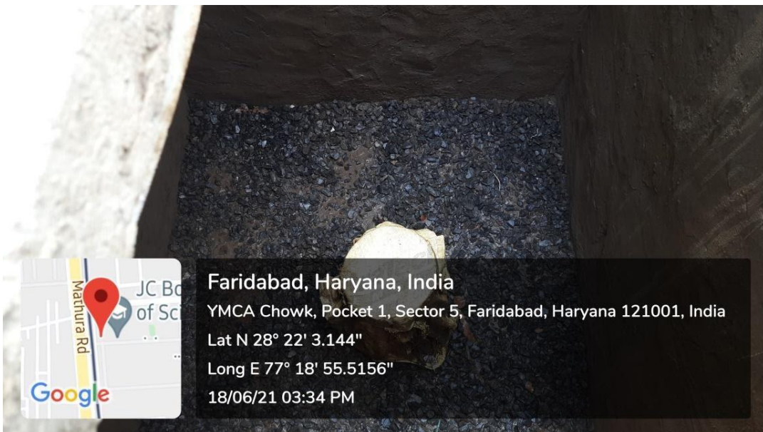
Image-08: Recharge Well at rear corner of Playground area
