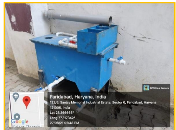
Effluent Treatment Plant behind C.V. Raman Block
