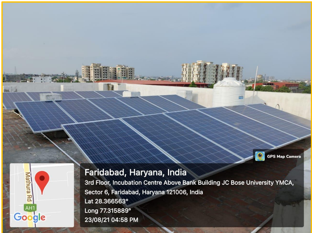
10 kWp Solar panels installed at roof-top of Community College Building
