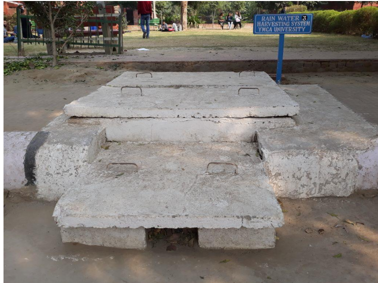
Rainwater Harvesting System at JCBUST, YMCA
