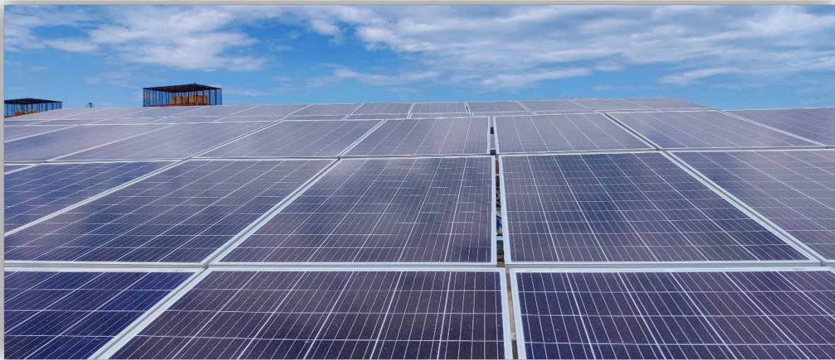
63 kW SOLAR PLANT (Actual Site)
